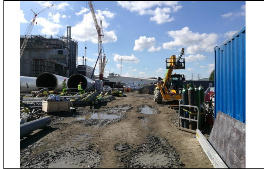
Photo 2 - General view of K3 construction laydown area. K3 is on the left hand side of the photo
